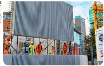
Precast concrete on-site lifting and install Assembly building C Bristol by AHMM & PCE Ltd
