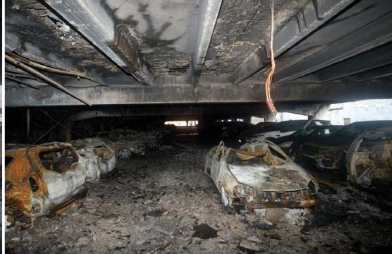
Above and below: From a structural stability point of view the Liverpool Echo Arena car park appears to have performed better than expected.
