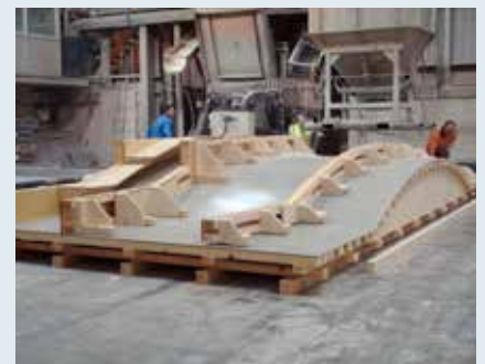
Above: The gently arching vaults weigh up to six tonnes Top: Each column is 3.1m high and 600mm in diameter
