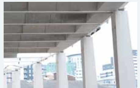
Above: The precast concrete columns taper in two directions, giving them a twisted appearance
