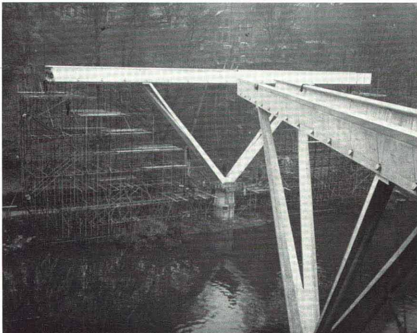
Below, left to right: Three stages in the rotation of a bridge half, from parallel with the shore to final joining.
